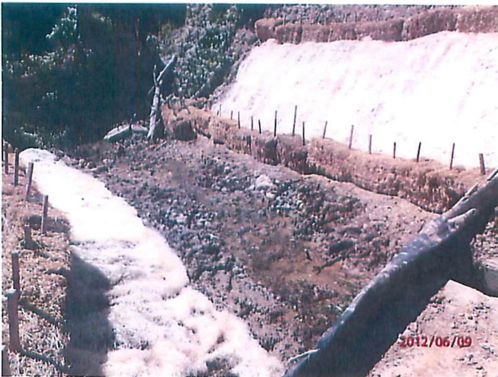
Photo 12. Stream crossing, post-blasting, on Tevebaugh Creek in Marion County with hay bales as primary E&S BMP.
