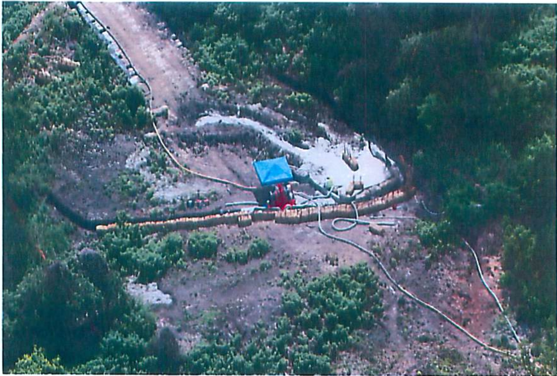
Photo 1. M3 inadvertent release of drilling mud on Monongahela River HDD (Horizontal Directional Drill) activity.
