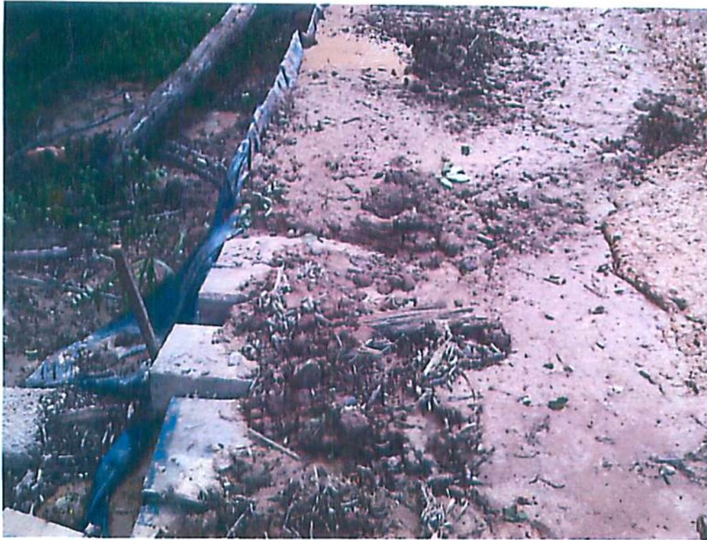
Photo 9. E&S BMPs in need of maintenance and/or repair on a stream crossing of Jake Run.
