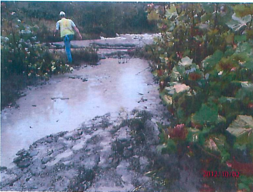
Photo 18. Expanded area influenced by inadvertent release of drilling mud into Dunkard Creek.
