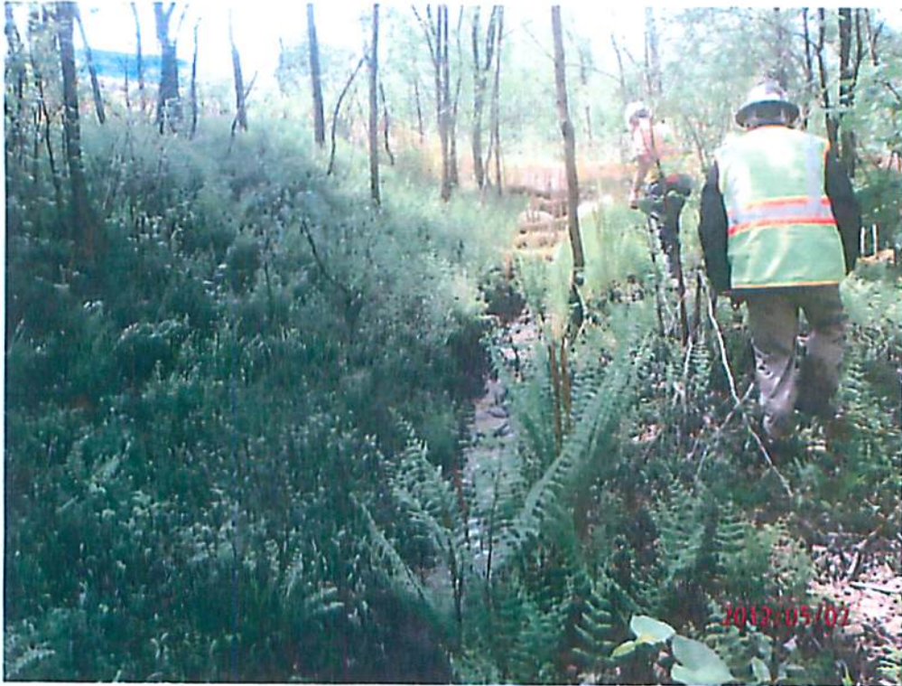
Photo 5. Site of inadvertent release of drilling mud from HDD activity into a UT of Monongahela River.
