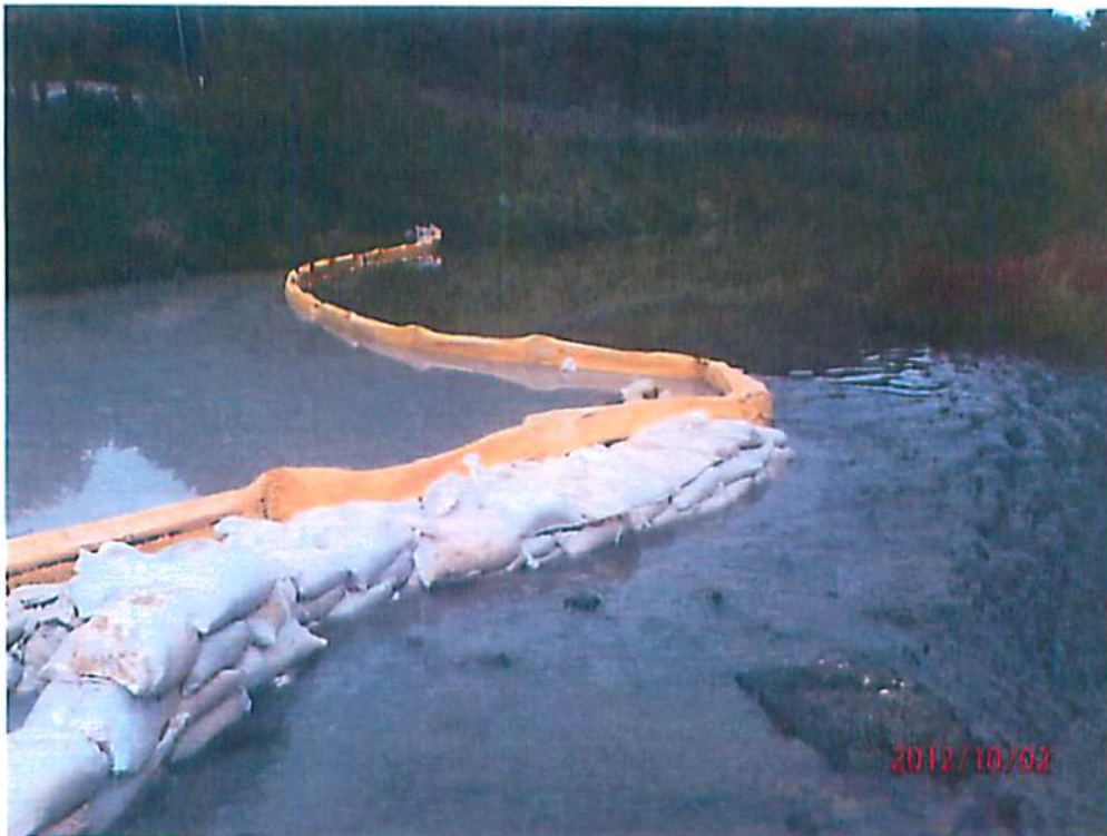
Photo 20. Containment around furthest-upstream inadvertent release into Dunkard Creek (showing turbidity curtain and sandbags).
