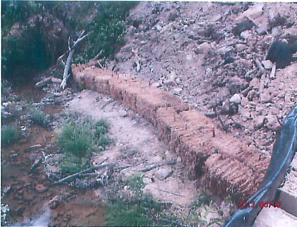
Photo 11. Use of hay bales as a primary E&S BMP (hay bales in need of maintenance and/or repair) and no bank stabilizer visible on Tevebaugh Creek in Marion County.
