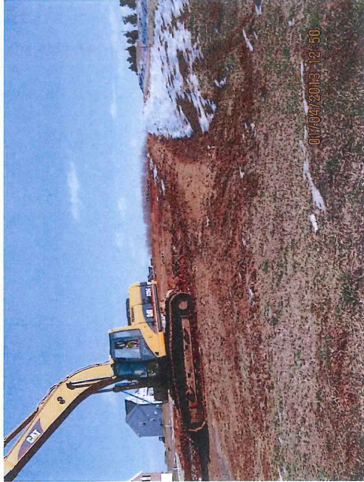
Charles Town: Unpermitted Land Disturbance
