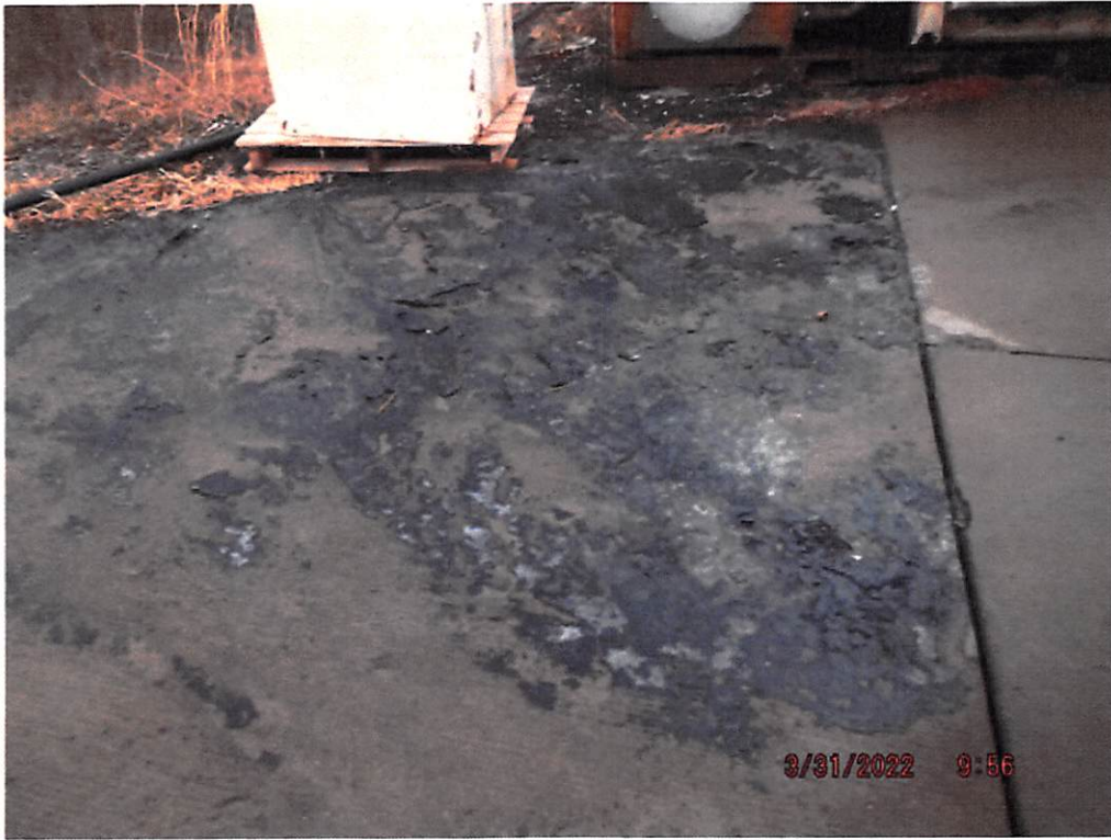
03/31/22 Burned and melted substance on concrete and on ground.
